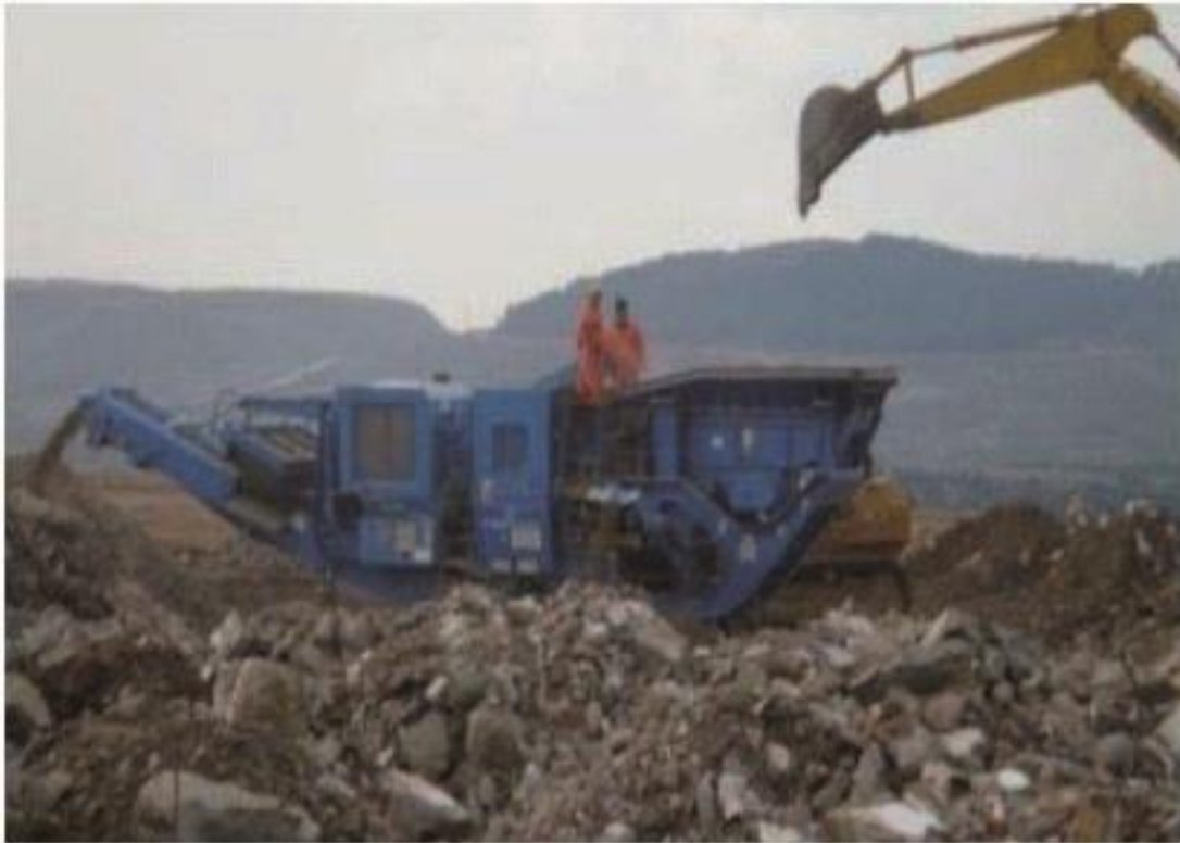
Figure 3.6 Demolition Waste Recycle Facility
