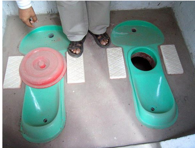
Figure 2.15: EcoSan waterless toilets
